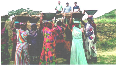
Photograph (2): Women workers actively participating in MGNREGA scheme in Aunta Panchyat of Mokama Block of Patna District.
